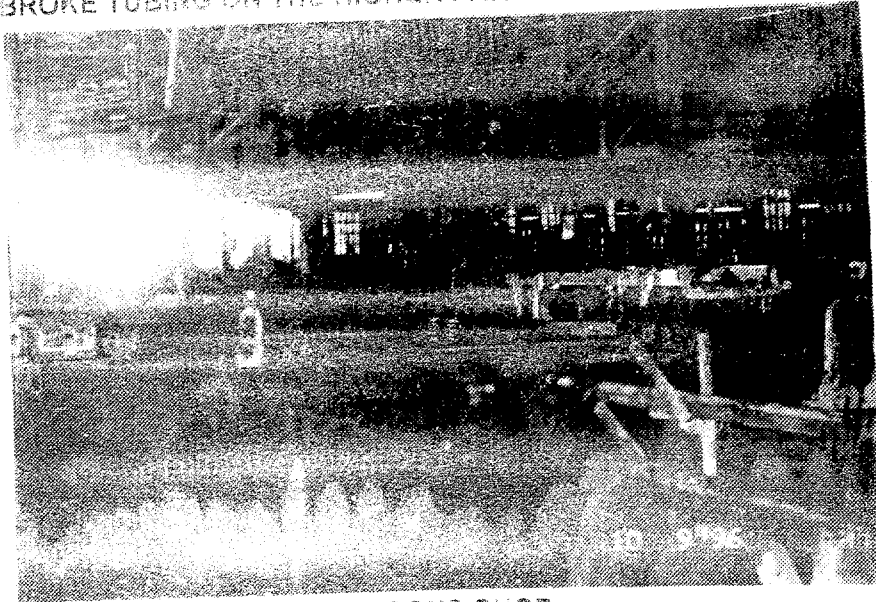
WAGONS SHOP (WATER ACCUMULATION ON FLOOR WITH OIL RESIDUE)
