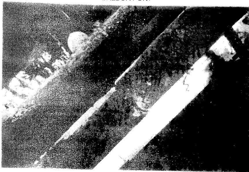
PIER 18, BROKEN WATER TUBES
